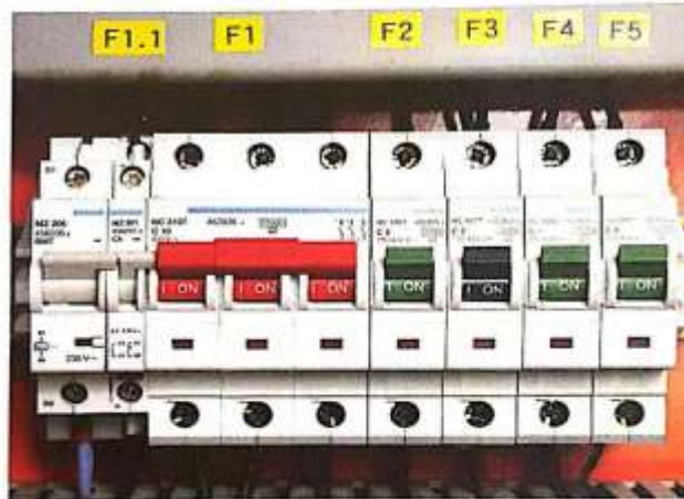
An electrical box
