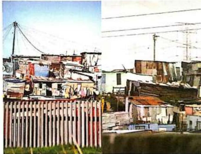
Illegal electrical connections in an informal settlement in Cape Town
